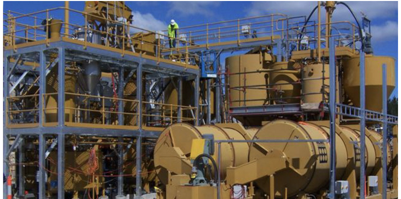
Figure 4: Continuous ILR at Ballarat Goldfields. This unit has been in operation for 15 years.
